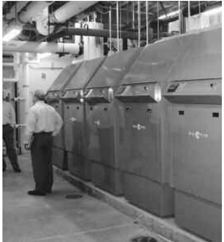
6 high tech, centrally located redundancy boilers saved $250,000 in original plumbing expenses.
